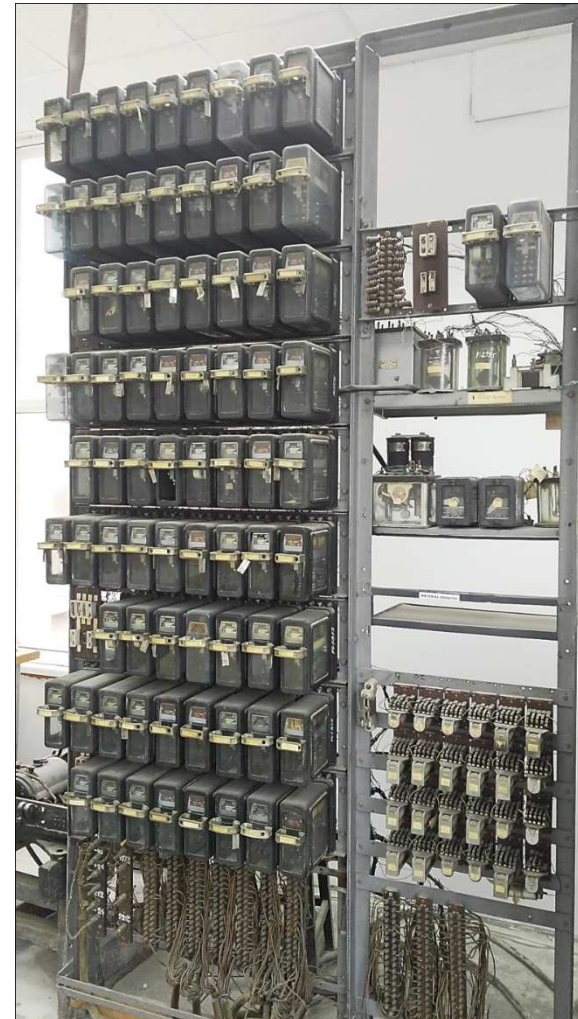
Example of relays frame
